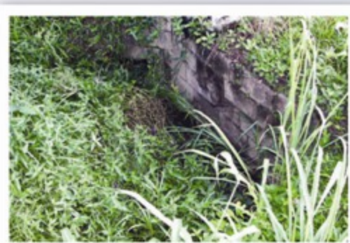
Captured at a site visit to a Regional Corporation complaint
